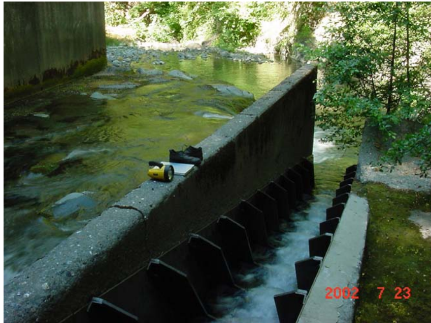
Figure 2.5. Fish ladder added to a culvert outlet to enhance fish passage.
