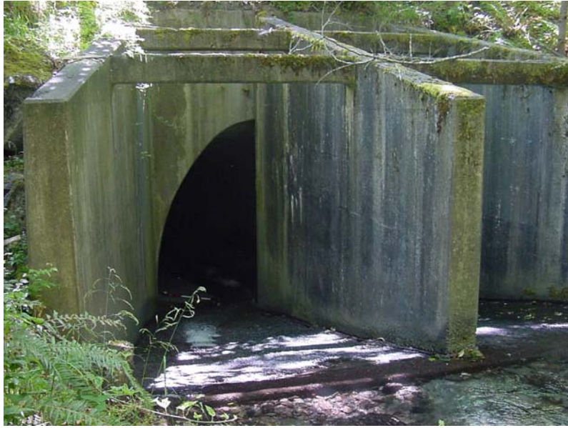
Figure 2.3. Concrete arch culvert with a concrete inlet apron and debris wall. If the apron has a steeper slope than the culvert, the apron may cause a velocity barrier to fish passage.
