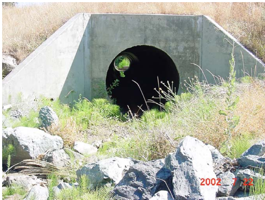
Figure 2.6. Wingwalls and headwalls guide flow into culverts and protect fill slopes from erosion.
