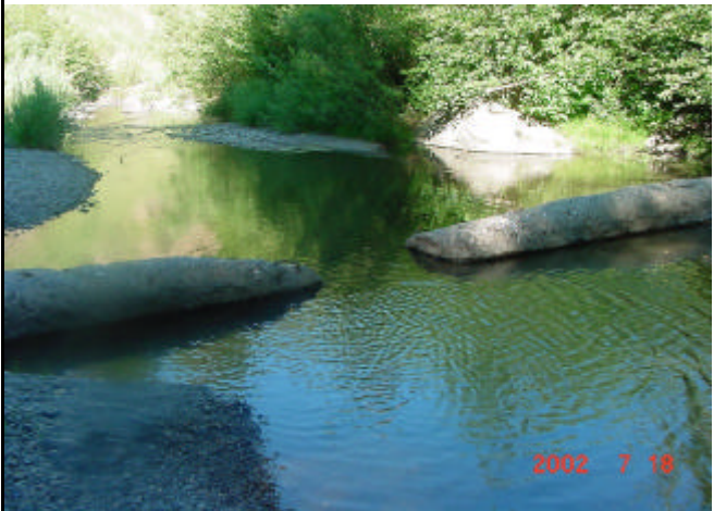
Outlet Apron and Notch
