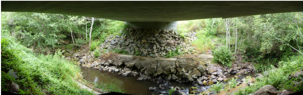
Figure 1. Undermined gunite false work and RSP material along right bank and in channel – Pre-treatment condition, 7/23/2013
