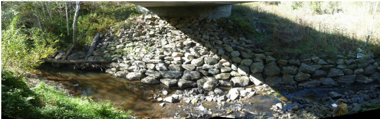
Figure 2. Newly placed RSP material and LWD feature placed along right bank – Post-treatment condition, 10/21/2015
