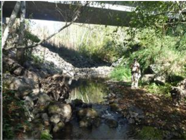
Figure 4. RSP removed from channel and LWD feature installed on right bank– (Post-treatment condition, 10/21/2015)
